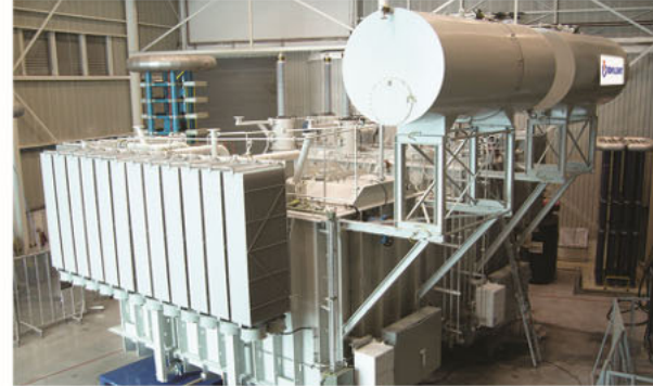
700 MVA, 240 kV, \pm 30^\circ in \pm 16 steps PST
